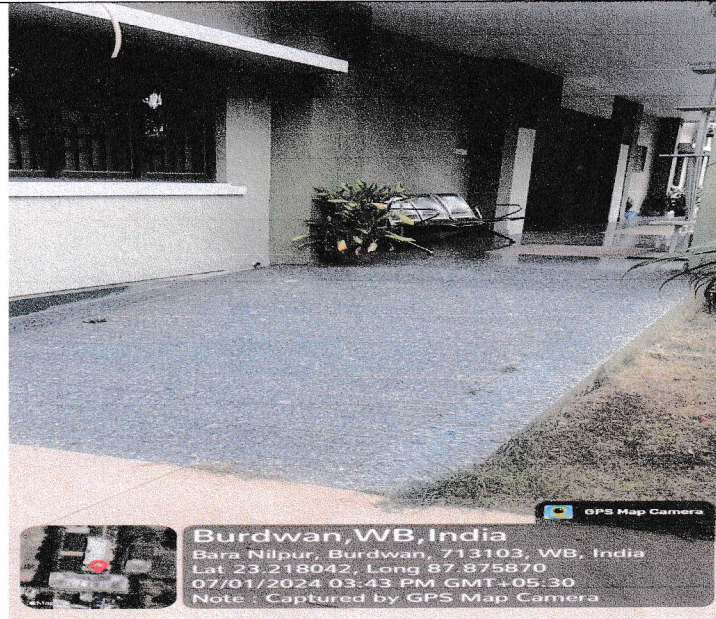
Disabled-Friendly Ramp at Academic Building
